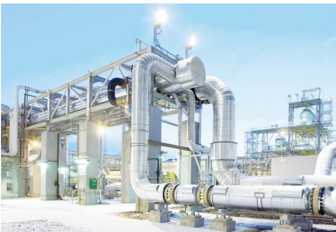
ABB provides systems and solutions for the automation and electrification of industrial processes across industries as diverse as oil and gas (pictured), pulp and paper, metals, minerals and mining, chemical and marine.
